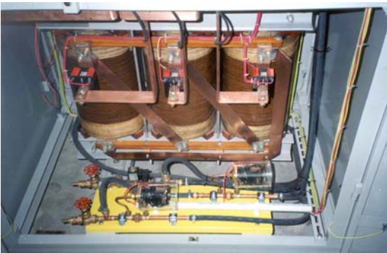
c) Power transformer with watercooling system
